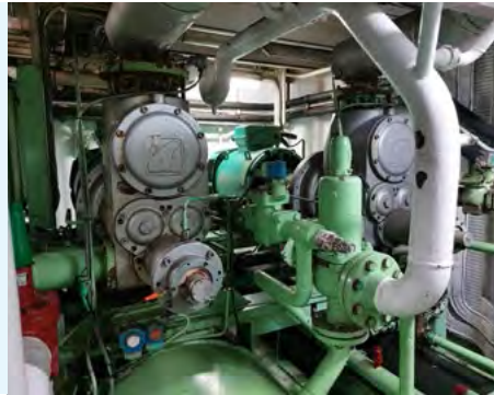
ABOVE The ammonia compressor, located in the refrigeration room, on board San Waitaki. 1
